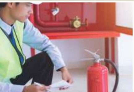
Fire Fighting System in Each Flat
